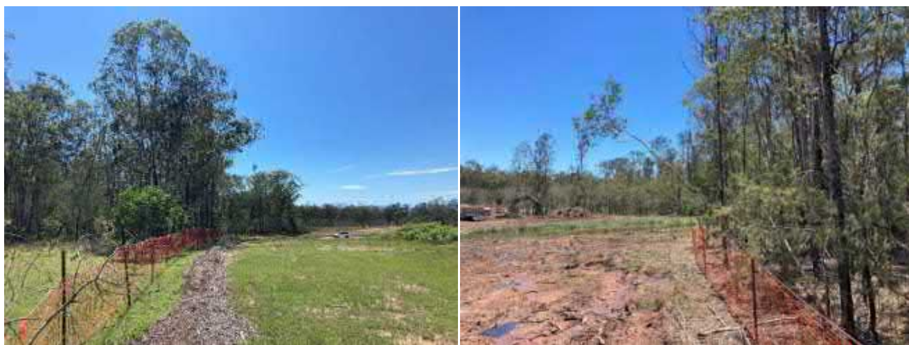
Photo Set 1: Maintained tree protection fencing and retained vegetation along Precinct 12 boundary (left) and ROL06 boundary (right) observed during annual site inspection and audit.
